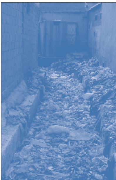
Before renovation: open drainage canal used as a refuse dump /26/
